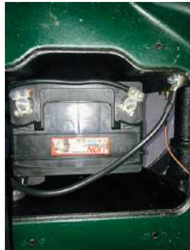
Single 12V battery in place
