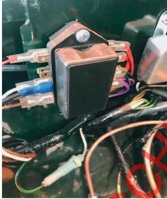
The small, neat fuse box housed 4 of the MGB fuses.
