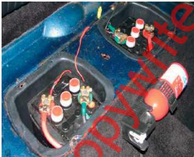
Twin 6V battery placement
